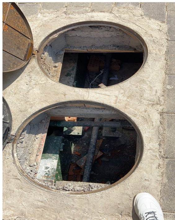
预留检修井盖
